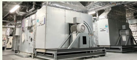
Air-conditioning equipment for which operating time was successfully reduced by revising how it is used
